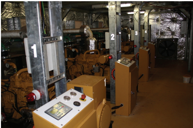
Fig. 19. Diesel Room at Eco Beach Resort
