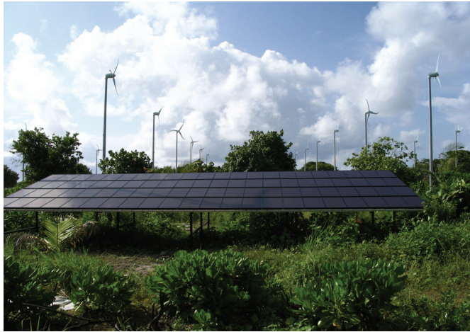
Fig. 13. Micro-wind farm and photovoltaic panels as installed in the Uligam island
