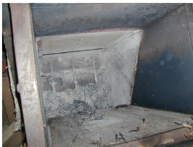
Fig. 9. The view of the furnace inside
