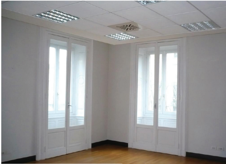
Fig. 5. Old lighting system with fluorescent lamps
